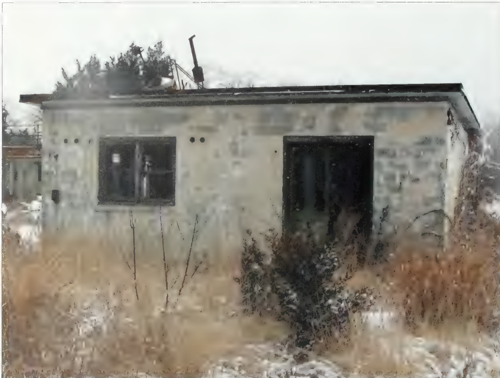
Figure 5.98. View looking southeast at the Generator Building (414), Control Area #1, NIKE radar site. The buildings and structures in the radar site show signs of deterioration in specific building materials that include metal, concrete block, and corrugated siding and roofing. Due to damaged windows and doors, the Generator Building lacks a closed building envelope exposing the interior to water and seasonal temperature fluctuations that advance deterioration (Olmsted Center, January 2009).
